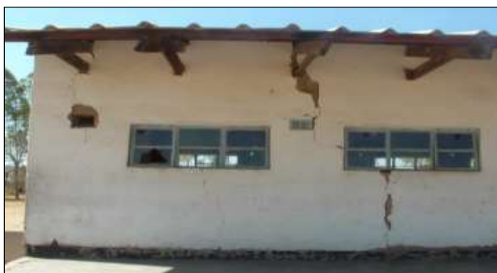
Plate 1: Cracks on a classroom block at Kowo School
